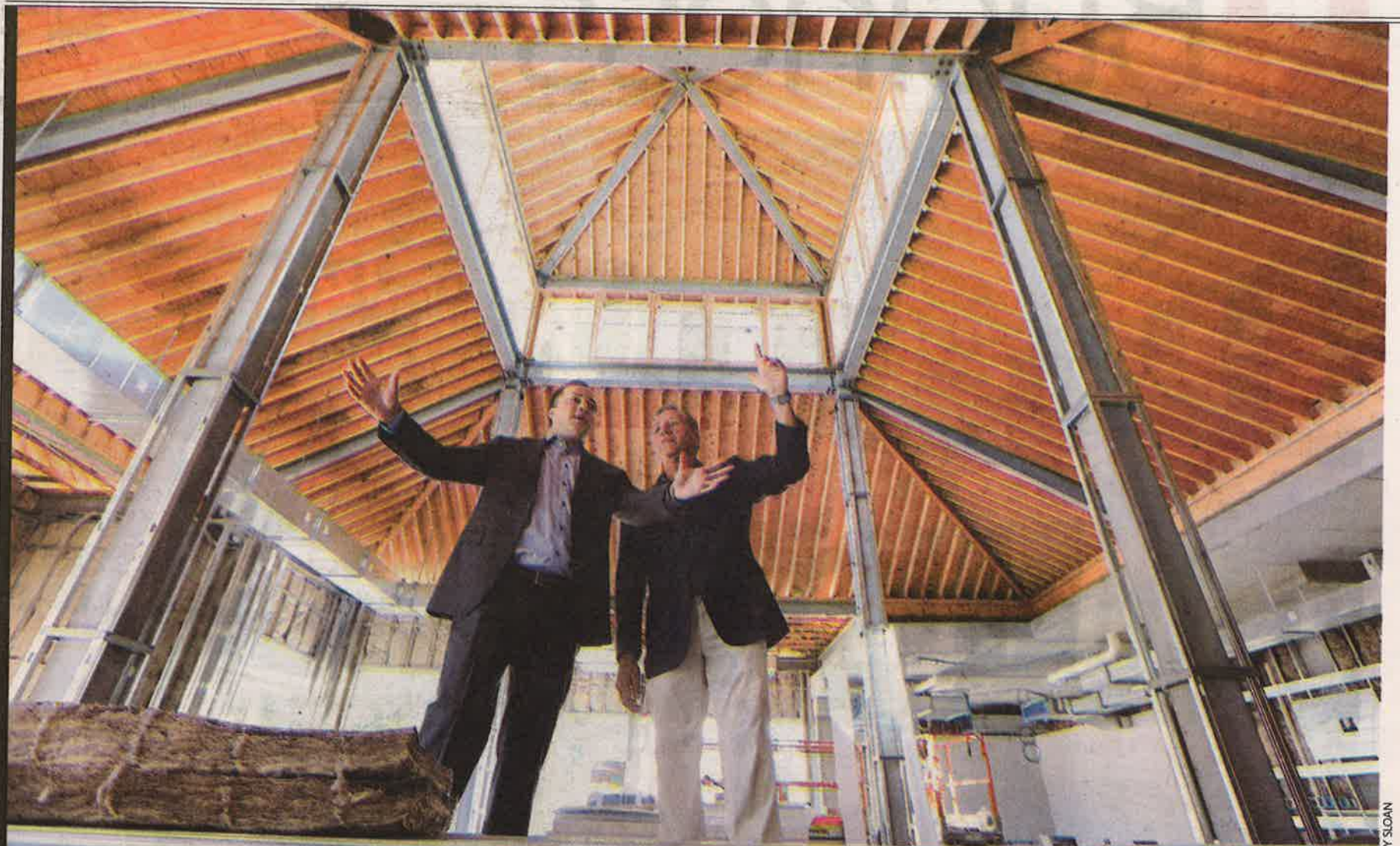
Co-developers Adam Levine, left, and Paul Amoruso discuss the progress of construction on the 165-room Hilton Garden Inn at 3 Harbor Park Dr. in Port Washington.
